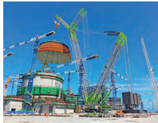
A team from the China Nuclear Industry Mechanical Engineering Co (CNME) hoisted the 487 tonne dome of the No. 1 generator unit at Zhangzhou Nuclear Power Plant in East China's Fujian Province. A 3,200 tonne capacity Zoomlion ZCC3200NP lattice boom crawler crane owned by CNME (10th place) made the lift
